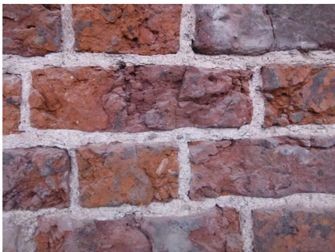
Figure 4 Detail of the brick bond in the façade walls. Photograph by Sara Pavia.
