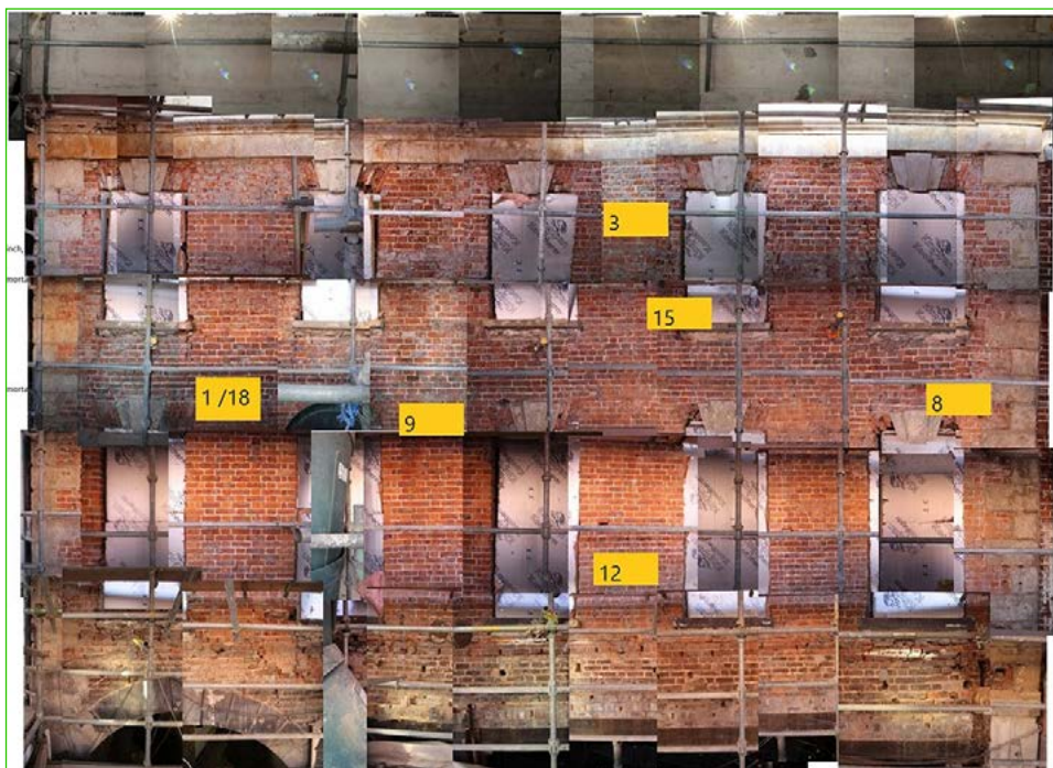
Figure 1 Fade Mansion during restoration work in 2018, showing the original brick fabric and the sampling. Published with the permission of Neil Crimmins of Cathal Crimmins Architects.
